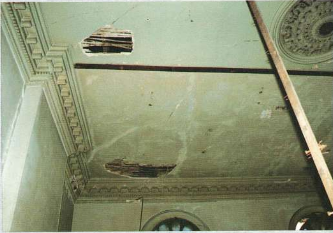
Ornamental lath and plaster ceiling requiring reinstatement
